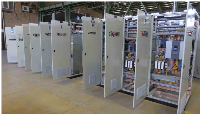
MCC Panel with VFD & Soft Starter
