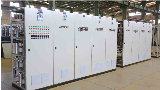
LV Capacitor Bank
